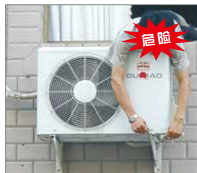
Very dangerous 非常危险
